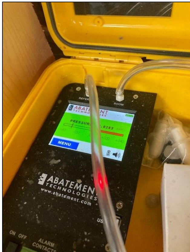
Figure 2.0: Adequate negative air pressure.
